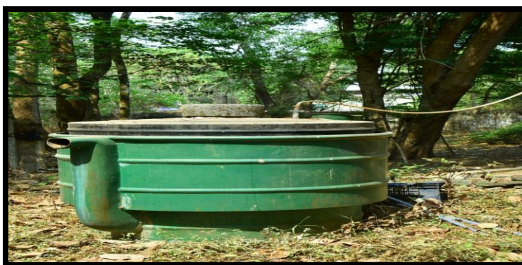
Biogas plant installed in MES Mampad College, Kerala.
